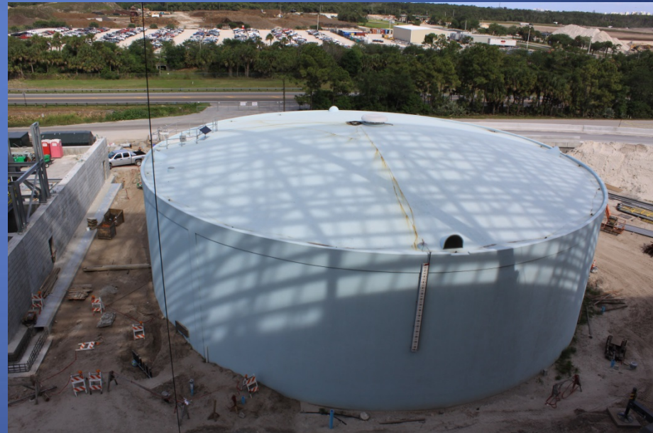
Two Million Gallon Rainwater Harvest Tank
