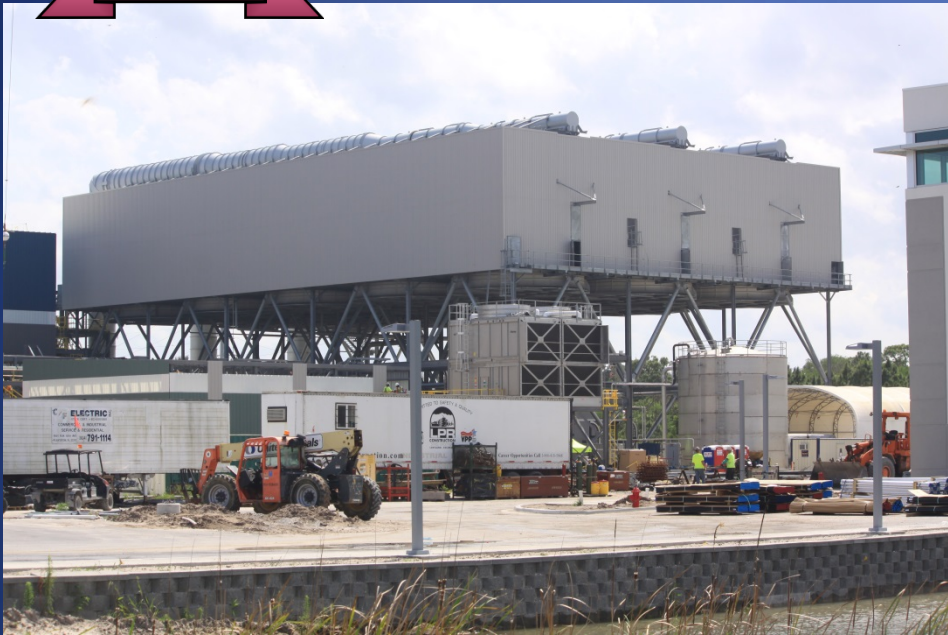
Air Cooled Condenser
