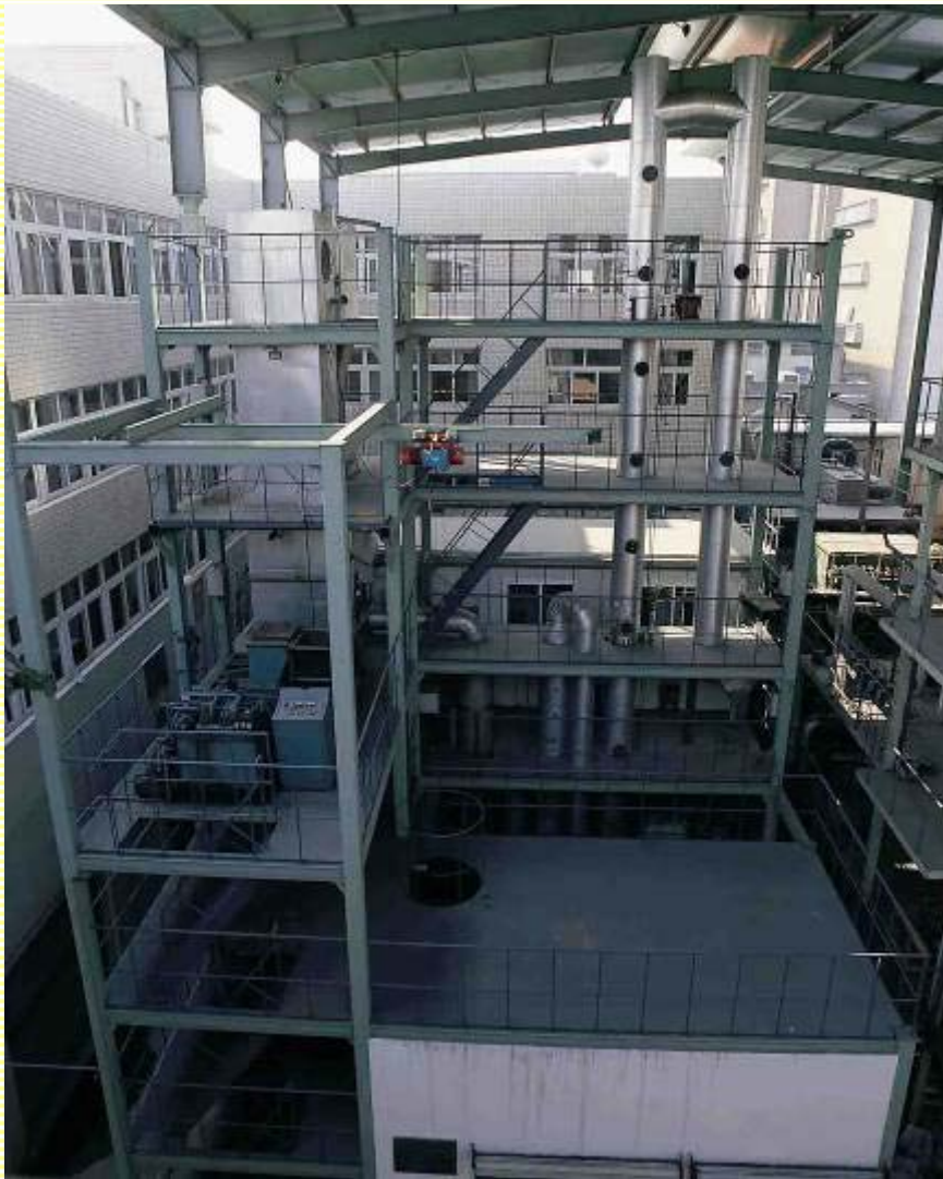
10t/d MSW test incineration system
