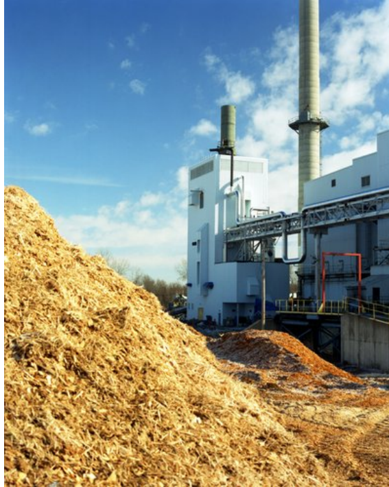
Figure 1-5. McNeil Generating Station in Burlington, Vermont, uses gasification technology to convert wood chips to power. Photo by Warren Gretz, NREL/PIX 04734
