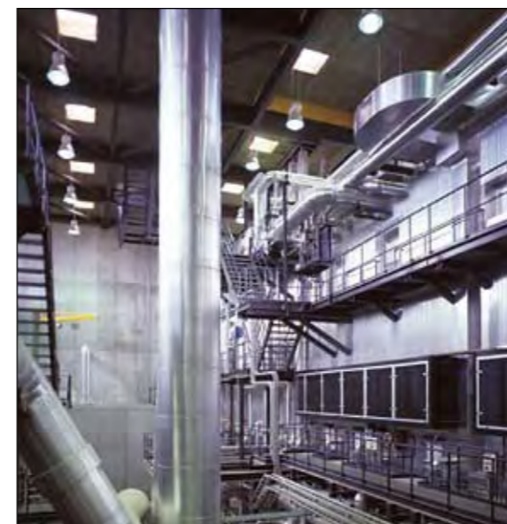
Interior of Svendborg CHP Plant.
