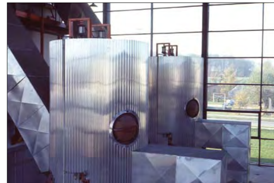
Interior of Nordforbrænding, 1969. In the front there are two multi-cyclone systems for the treatment of flue gases. In the mid-70s, electrostatic precipitators replaced the multi-cyclones, and in 1987 completely new, dry flue gas treatment systems with lime reactors and bag house filters were installed.
