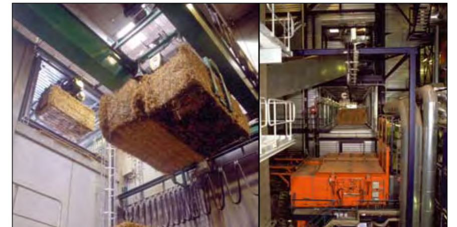
Conveyors and feeding of straw at Måbjergværket.
