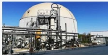
Dairy Feeds Biogas Plant With Whey
