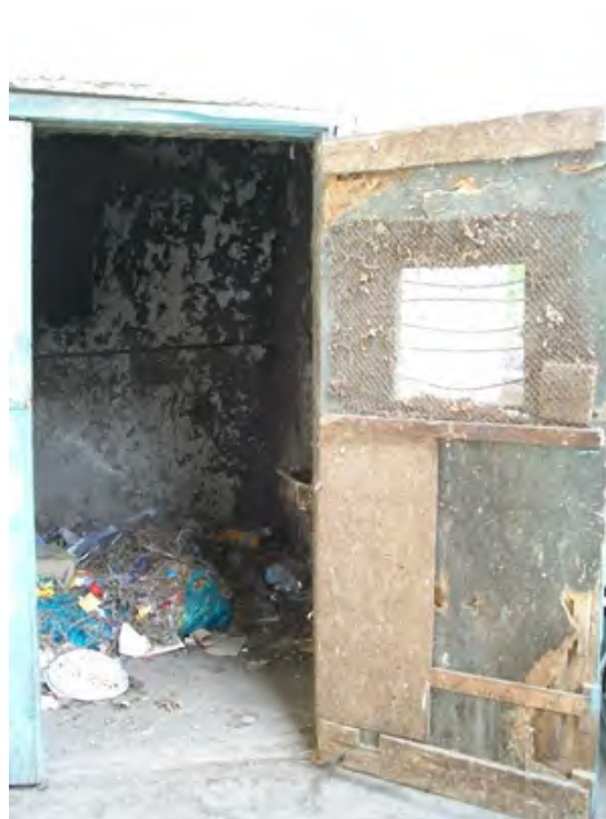
Figure 32: Waste Collection Point in Multi-Storey Building/Waste Chutes
