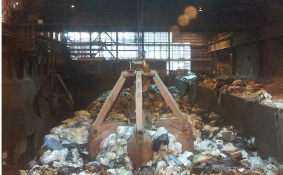
Figure 25 – A claw crane at Covanta's Essex plant taking MSW from the refuse pit, Newark, NJ.
