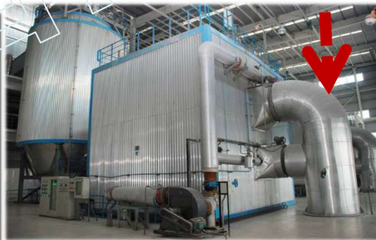
烟气净化 Flue gas purification system
