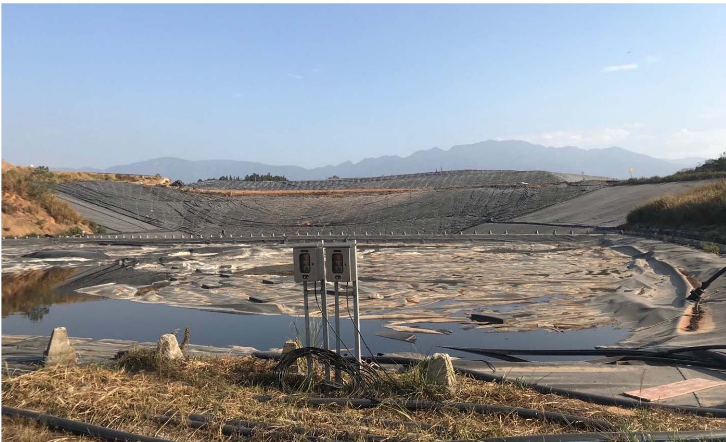
Landfill Leachate collection system (Jiujiang city, Jiangxi Province, China)
