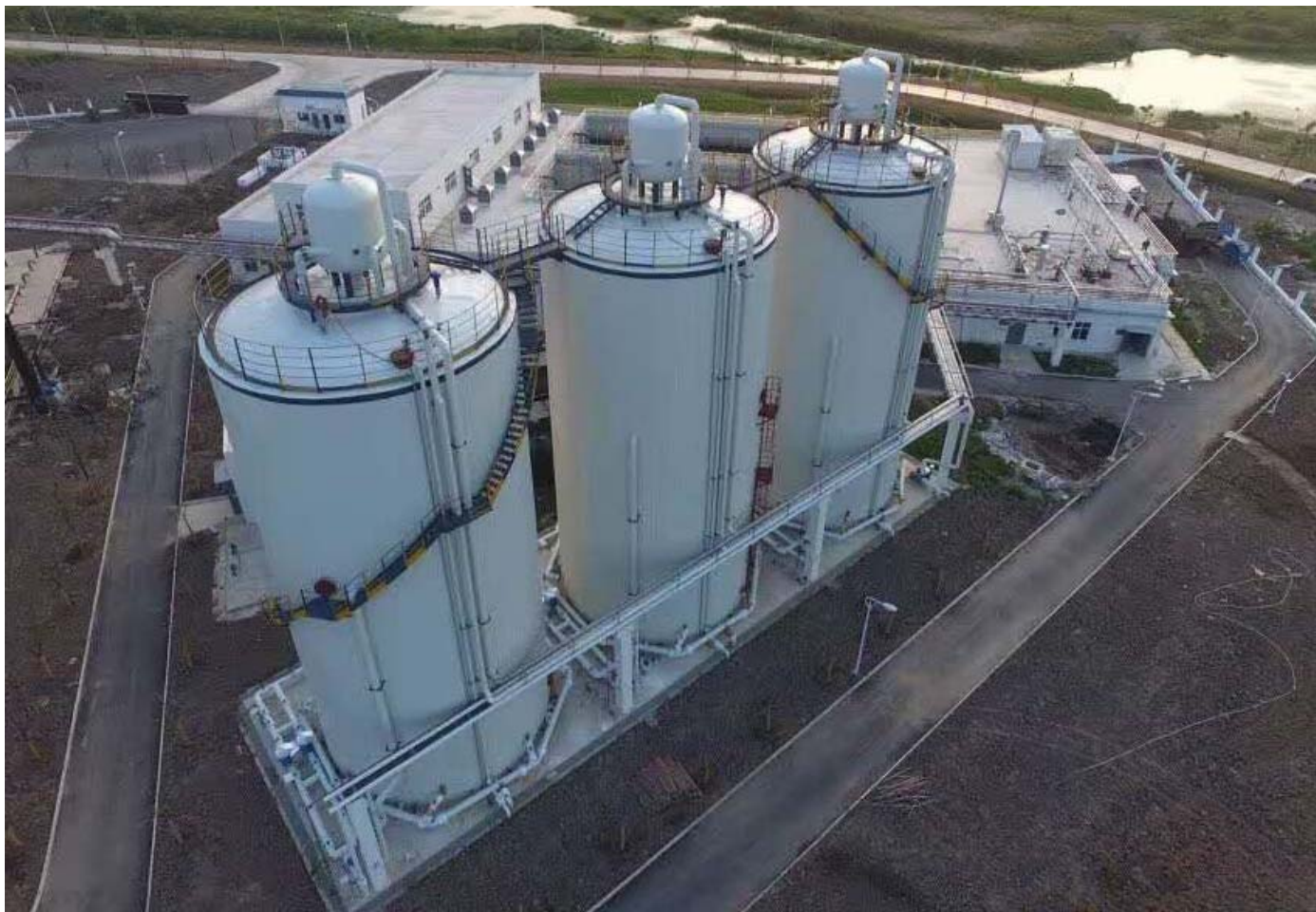
Leachate treatment in Wujiang waste-to-energy plant of EB
