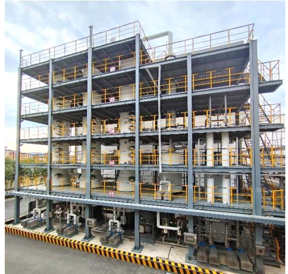
Application in leachate treatment
