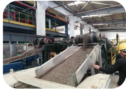
Bottom ash sorting equipment
