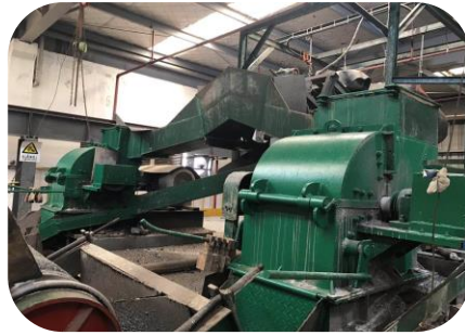
Bottom ash breaking equipment
