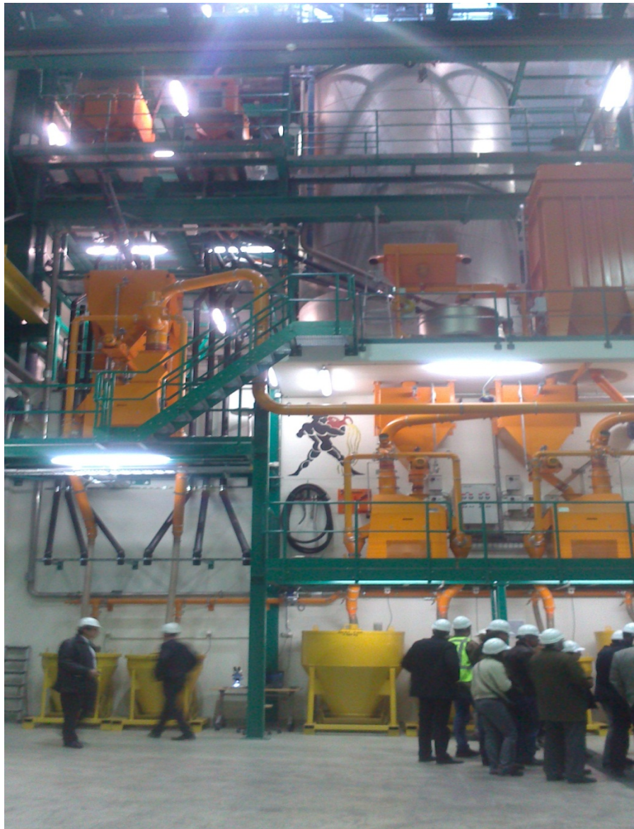
Figure 3. IBA dry discharge technology in Hinwil, Zurich 8
