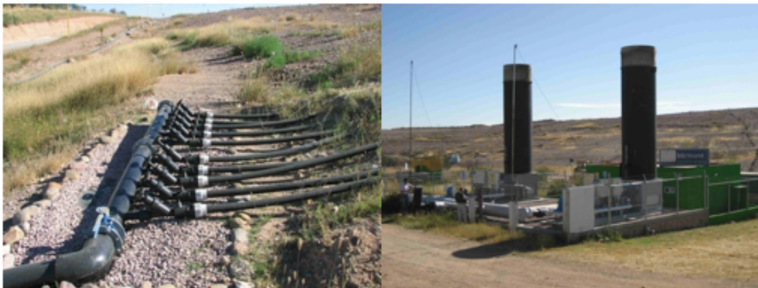
Figure 27: San Nicolas de Arriba sanitary landfill installations (M2M, 2009)
