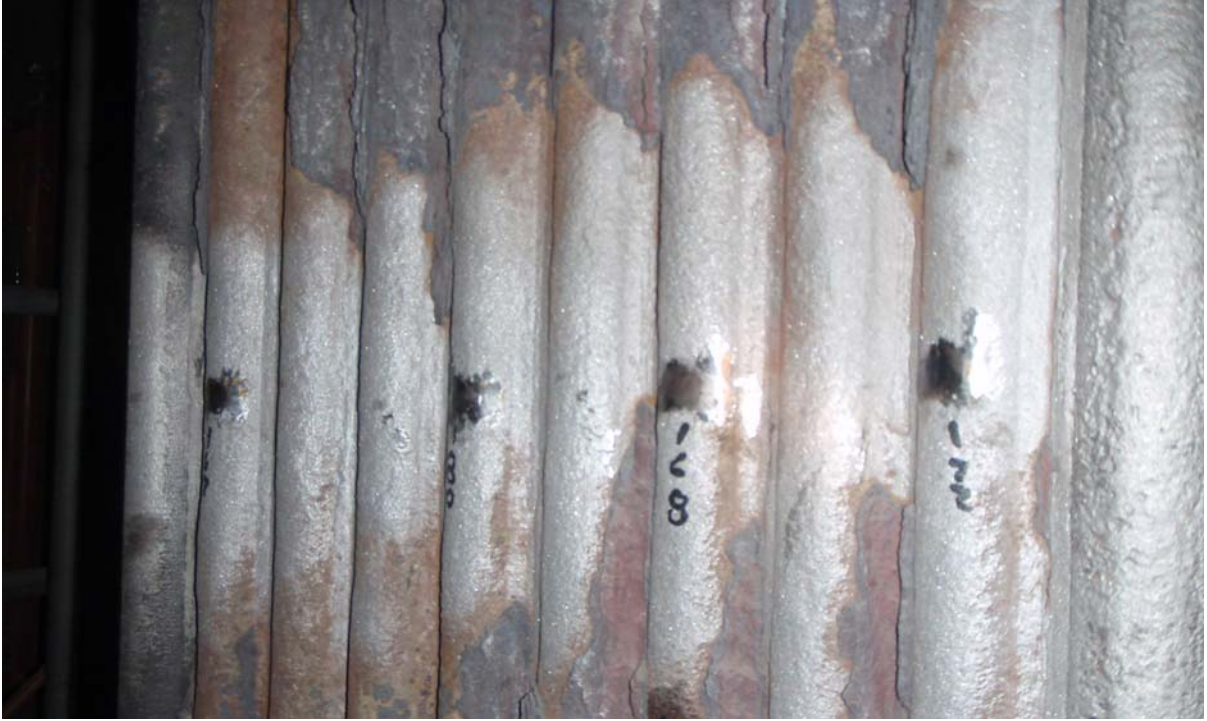
Figure 11. Panel 3-7 (one of five non-trials) with Inconel 625 weld overlay for the lead and trail tubes and 8 unprotected SA-213T22 tubes in between after one year of operation (with tube wall thickness readings).
