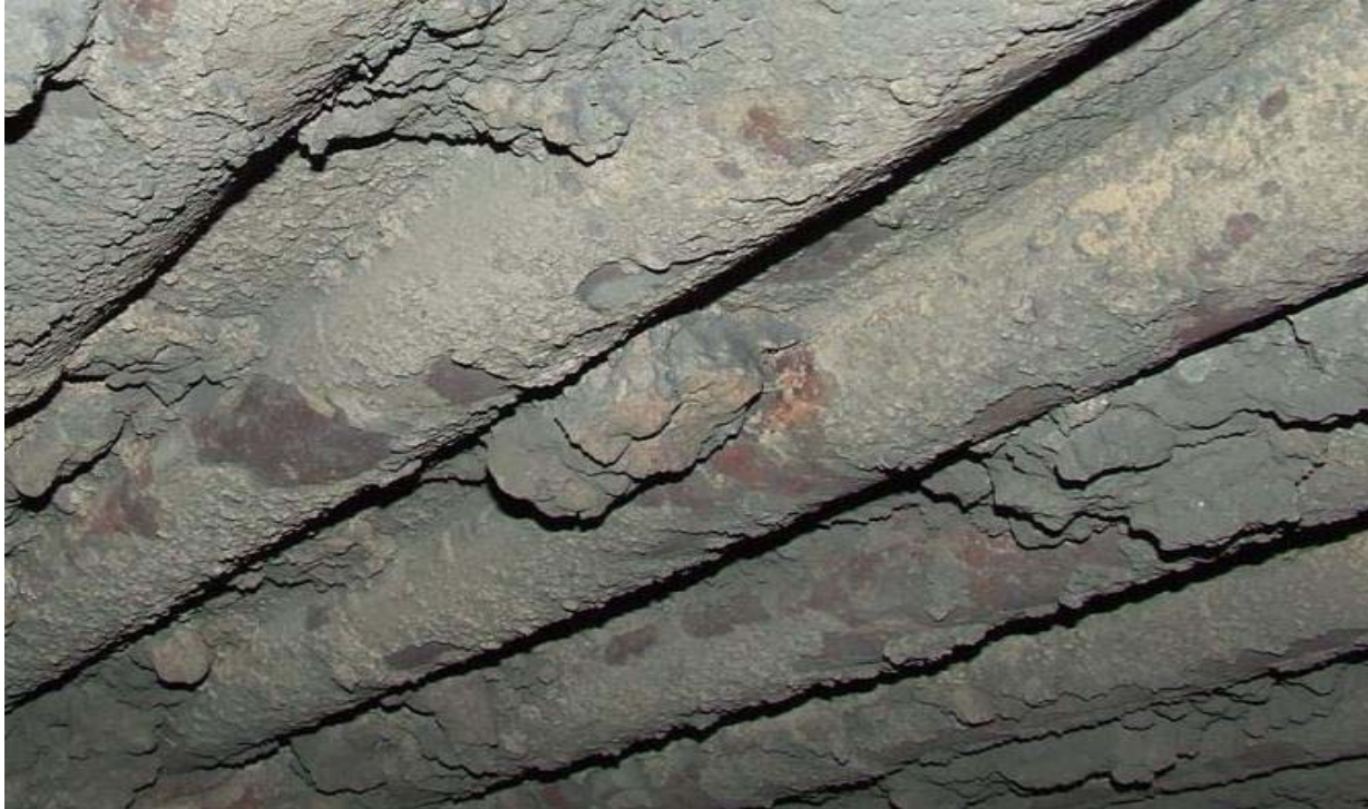
Figure 1. Roof waterwall area covered by slag before it was removed prior to AmStar’s cladding activities.
