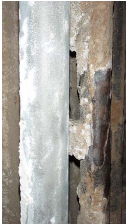
Figure 8. AmStar 888® cladding on left tube after 3.5 years of operation in comparison to an unprotected adjacent tube being in service for only 18 months
