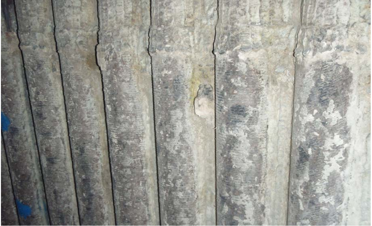
Figure 7. Visual inspection illustrating that no thinning or delamination occurred where the cladding was applied over old weld overlay.
