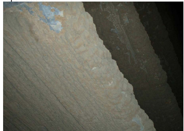
Figure 9b – platen superheaters EfW plant Naples/Italy, status November 2009
