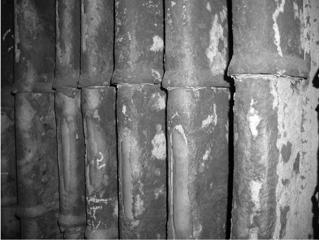
FIGURE 1- INSTALLED HIGH TEMPERATURE SUPERHEAT SHIELDS AFTER 1 YEAR OF OPERATION
