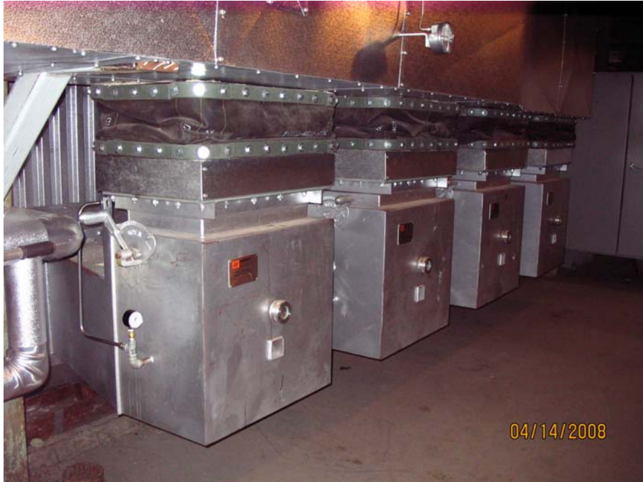
PHOTO 1. POST-UPGRADE OFA NOZZLES ON THE LEFT SIDE WALL
