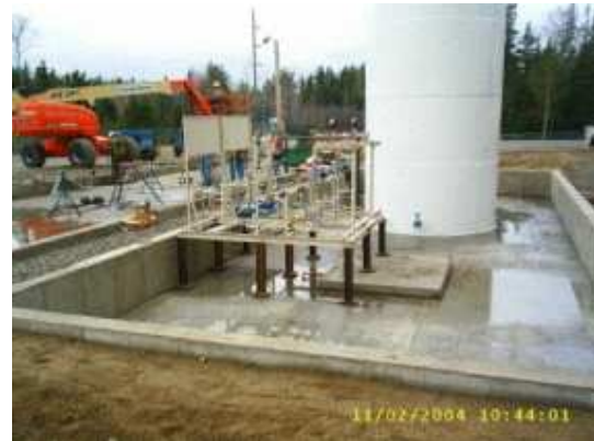
FIGURE 5: AMMONIA SKID/STORAGE TANK -50 MW RSCR
