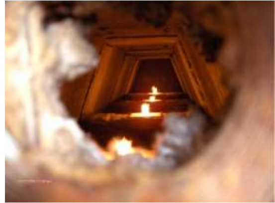
FIGURE 4: PHOTO OF RSCR SYSTEM BURNERS IN OPERATION
