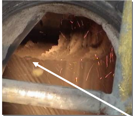
Figure 6: Deposits Removed As Far As 20 Feet From Lance Tube Exit – Non-Line of Site Cleaning
