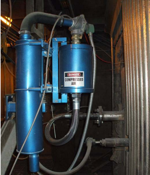
Acoustic Sound Generator (ASG) Unit 2 Covanta Hempstead, NY
