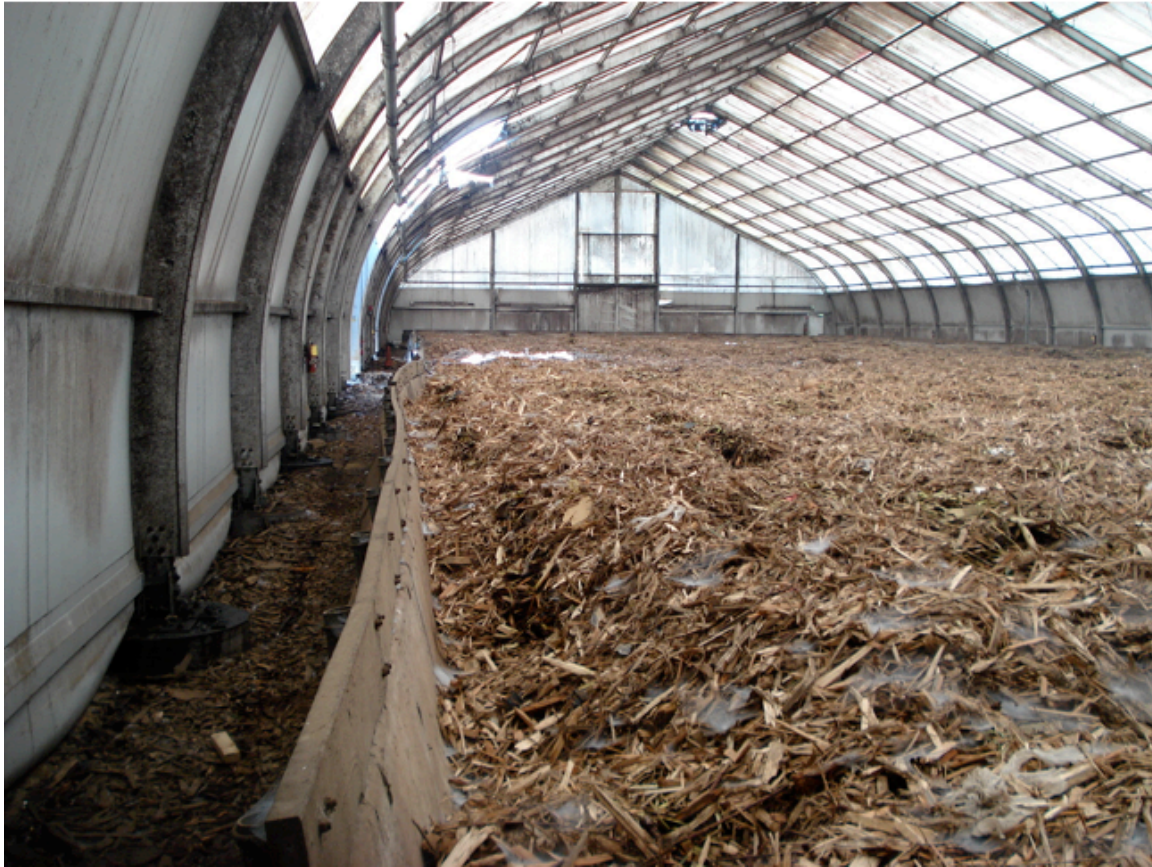
Figure 21: Biofilter system with a 20,000 ft 2 area of woodchips that clean the odorous air from the composting processes.
