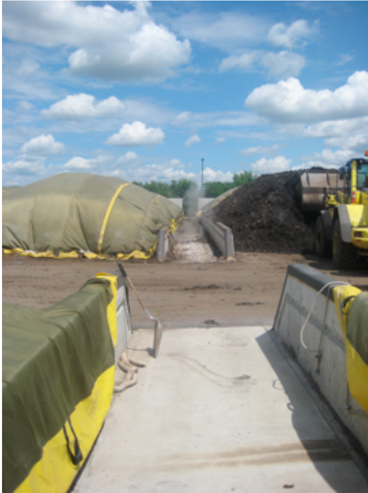
Figure 14: The composting area with the vertical walls to which the covers are attached with rubber ropes. On the right, a pile is being transported from one windrow to the area.
