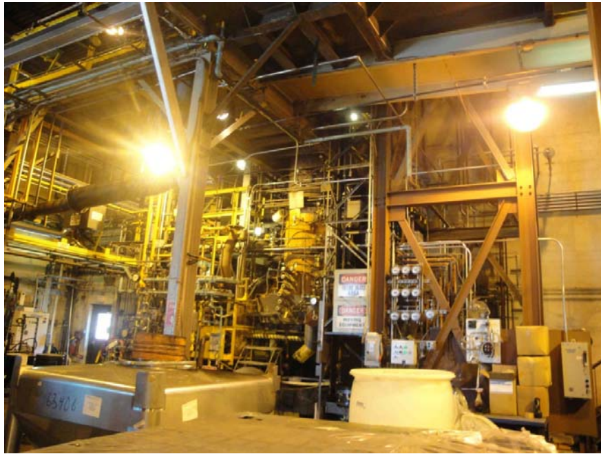
Figure 39. Overall view: gasifier, quenching system
