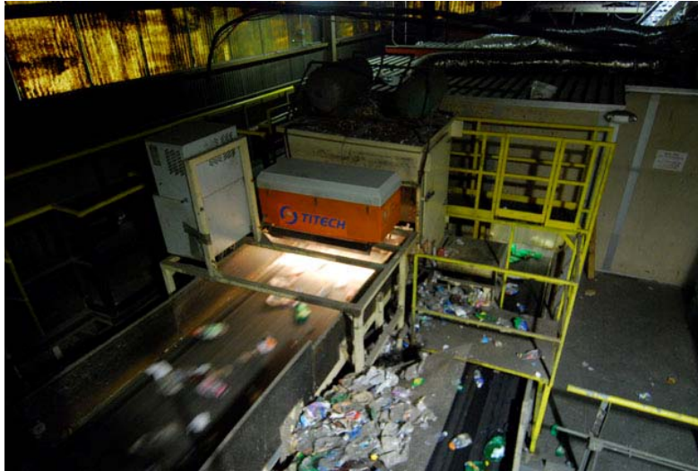
Figure 6.2 : One of ten Ti-Tech NIR scanners in use at Raleigh Plastics
