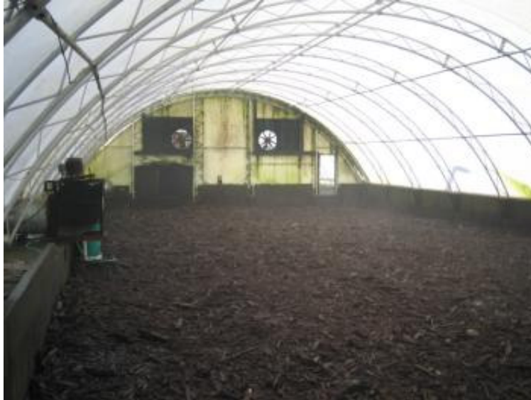
Figure 20 Biofilter on the Newmarket facility installed as part of the Remediation Plan in 2007 (photo by L. Arsova)
