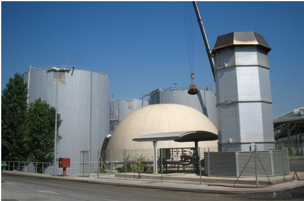
Figure 28 Anaerobic digestion reactors, gas tank and the gas stack on the site of Ecopark 2 (photo by L. Arsova)
