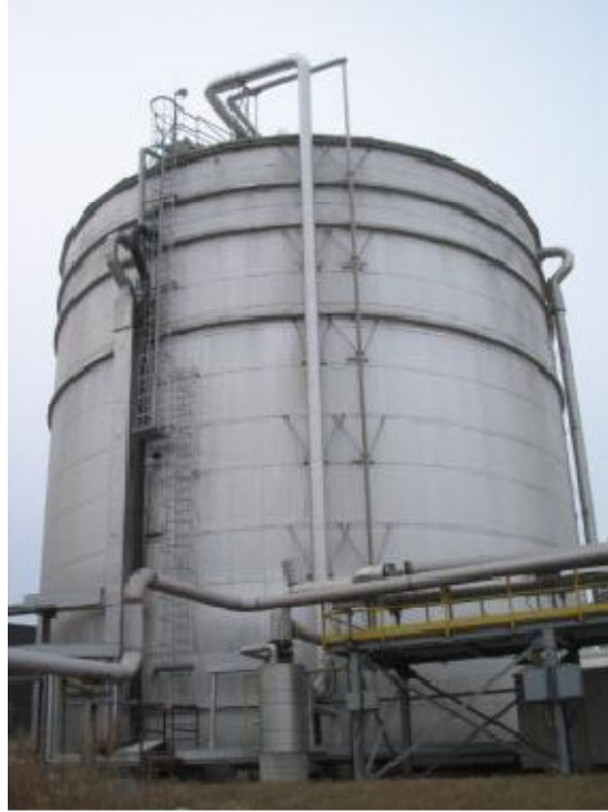
Figure 13 Anaerobic digester on the Dufferin AD plant
