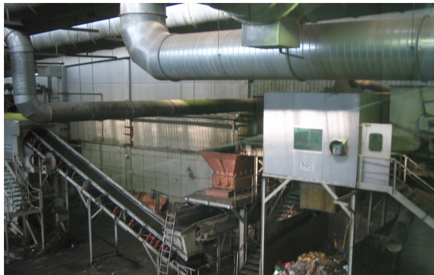
Figure 27 Sorting cabin, bag breaker and tromell at the beginning of the pretreatment of the SSO fraction (photo by L. Arsova)
