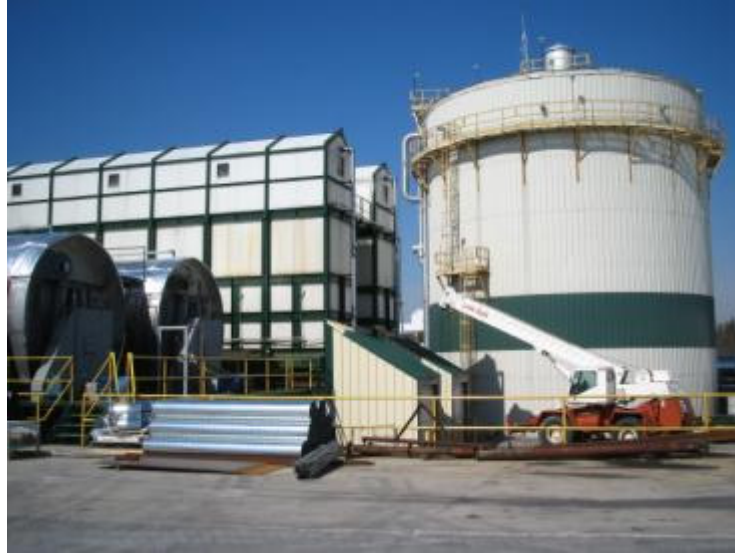
Figure 18 Anaerobic digester and aerobic VCU at the Newmarket plant
