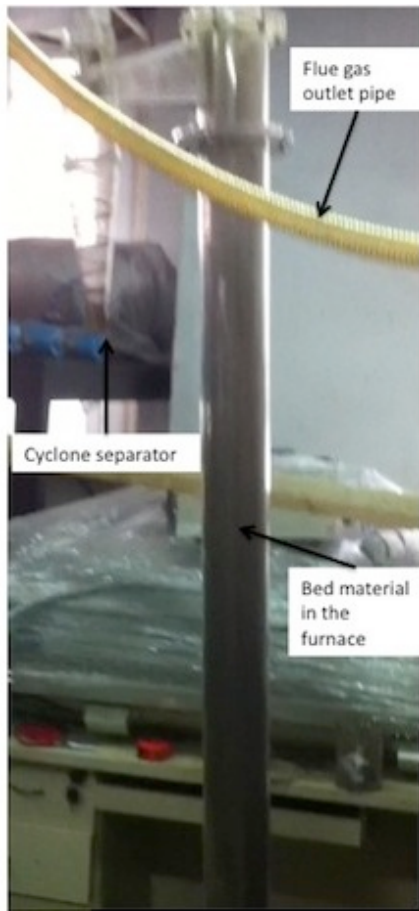
Figure 24: Photo of the empty furnace and of cyclone separators
