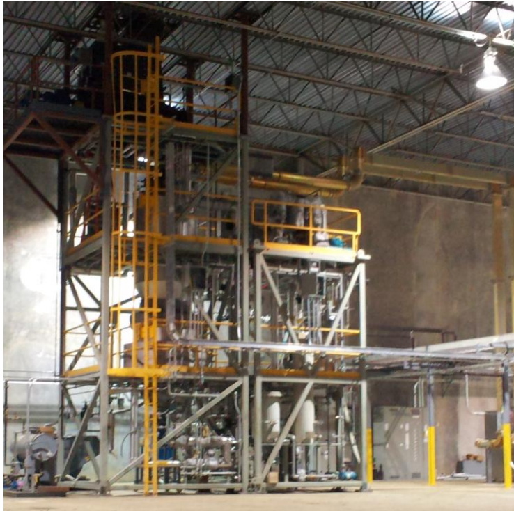
Figure 16: Climax Global Energy Inc.'s Commercial Unit Source: Climax Global Energy Inc. (2013)
