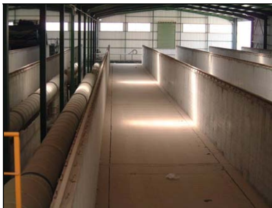
Figure 4.46 Channels in the composting unit (21) .
