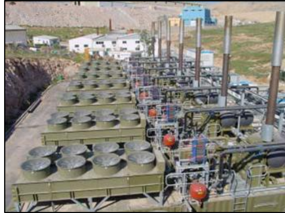
Figure 4.59 Mobile energy production modules (50) .
