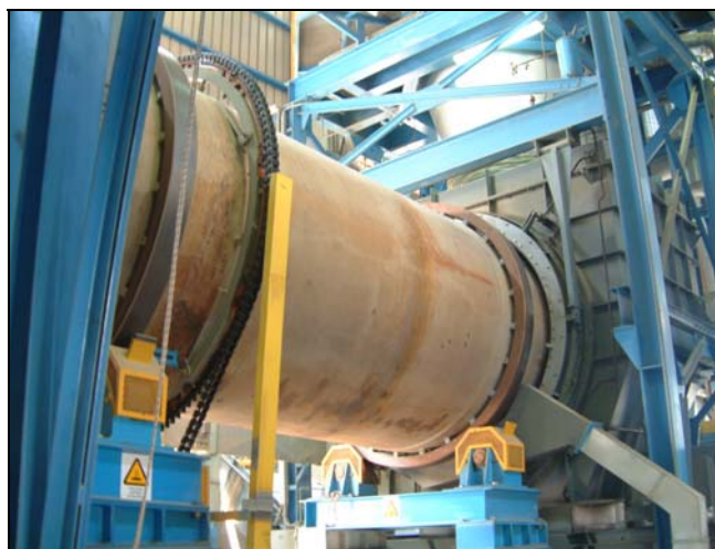
Figure 4.49 Rotary kiln of the MWI (21) .
