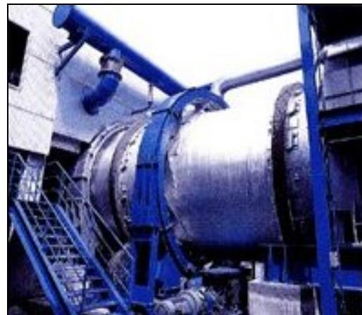
Figure 2.16 View of a rotary kiln (162) .
