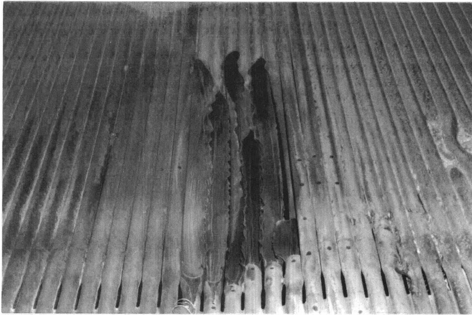
FIG. 3 UNIT 3 TUBE FAILURES, JUNE 1990
