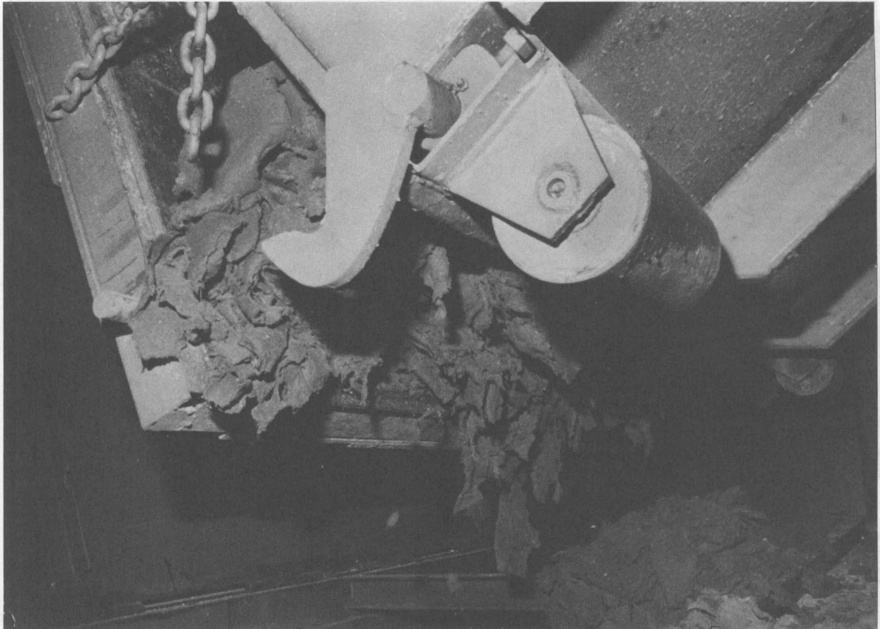
FIG. 10 VIEW OF SLUDGE EXITING ROLL-OFF CONTAINER INTO THE SLUDGE BIN
