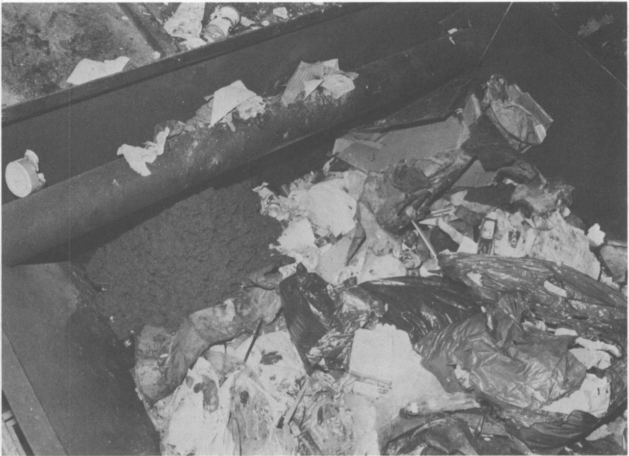
FIG. 12 VIEW OF DELIVERY PIPE AND SLUDGE IN THE FEED HOPPER OF THE INCINERATOR
