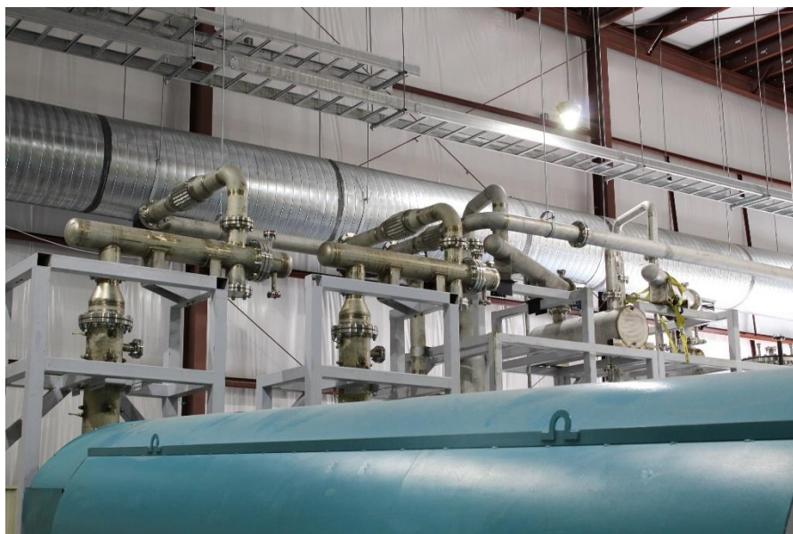
Fig. 1 Full-scale plant of Renewlogy & Sustane Technologies.
