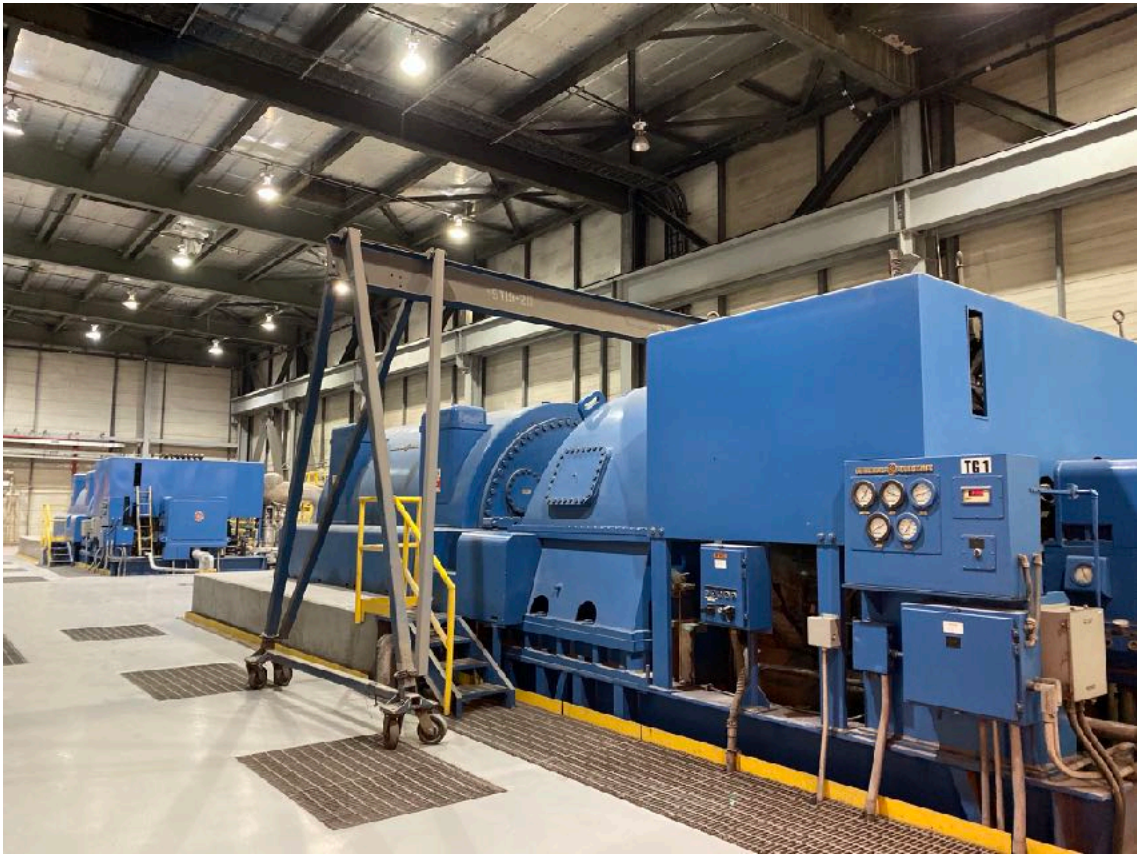
Figure 8: Energy generation, two General Electric 35 megawatt units. 9
