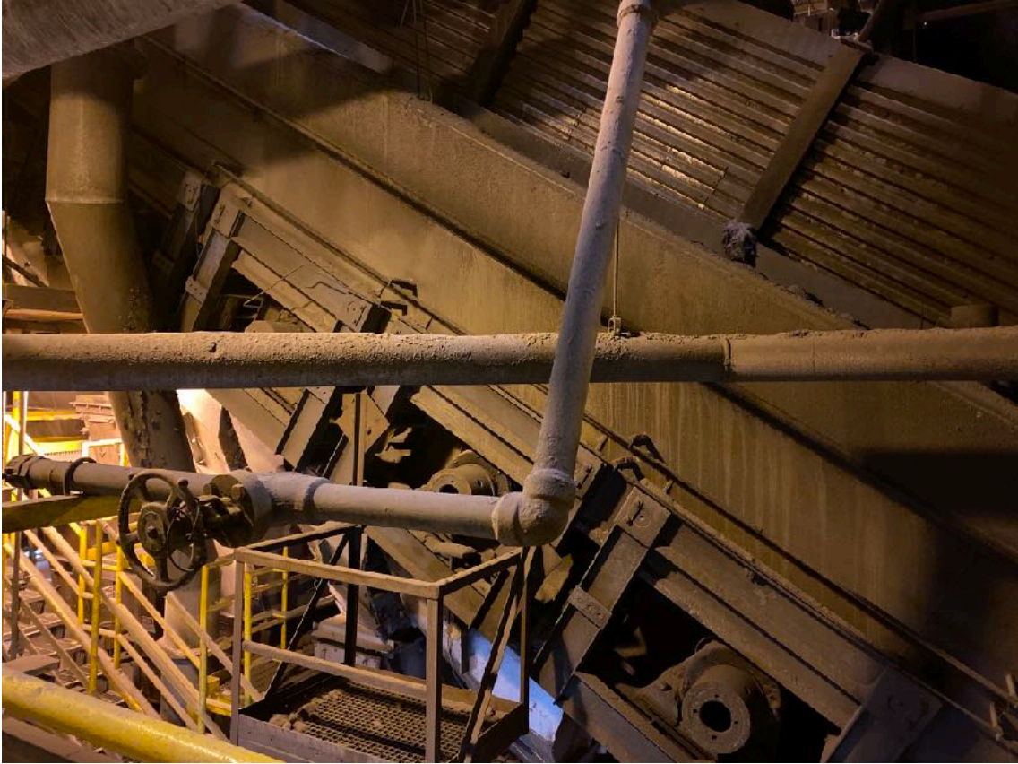
Figure 7: Bottom of the Roller Grate System.
