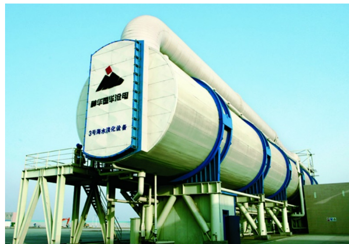
Figure 26 Guohua Cangdong Power Plant Desalination Facility (25,000t/d)
